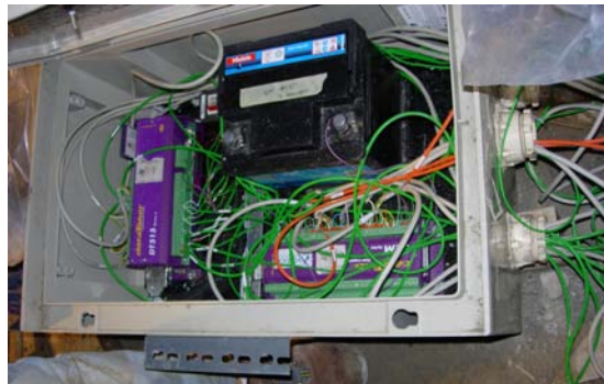
Figure 6.30: Datalogger system installed in the gallery
